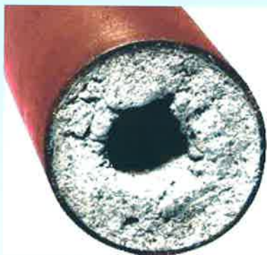
Limescale build-up in pipework
